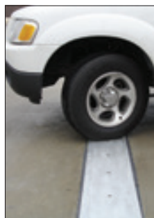
Watertightness is assured at the traffic surface negating the need for ineffective moisture barriers and secondary gutters.
