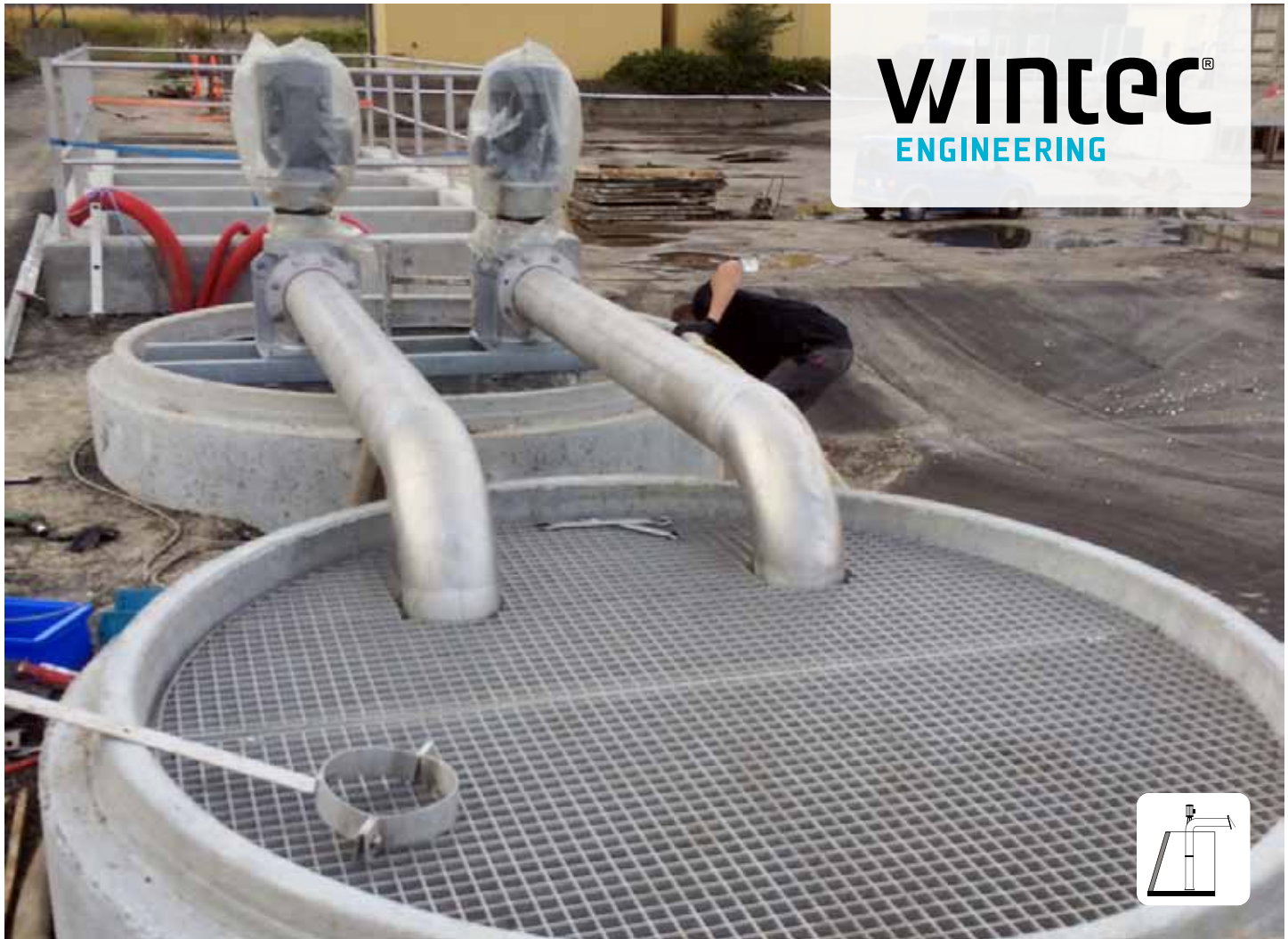
Pumpestation m. VENERONI propelpumper 400 l/sek.
