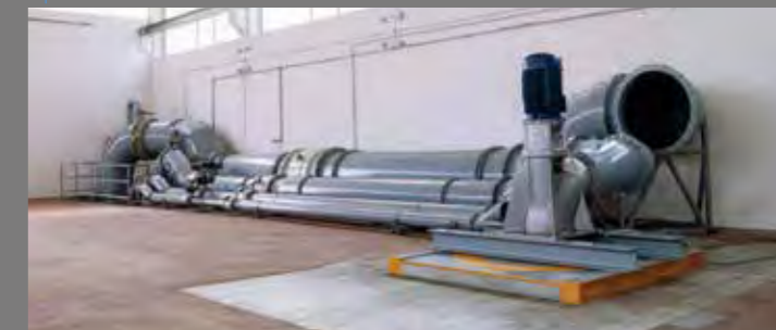
Sala prove Testing Room
