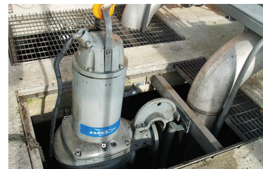
3000 Series Pump Installed
