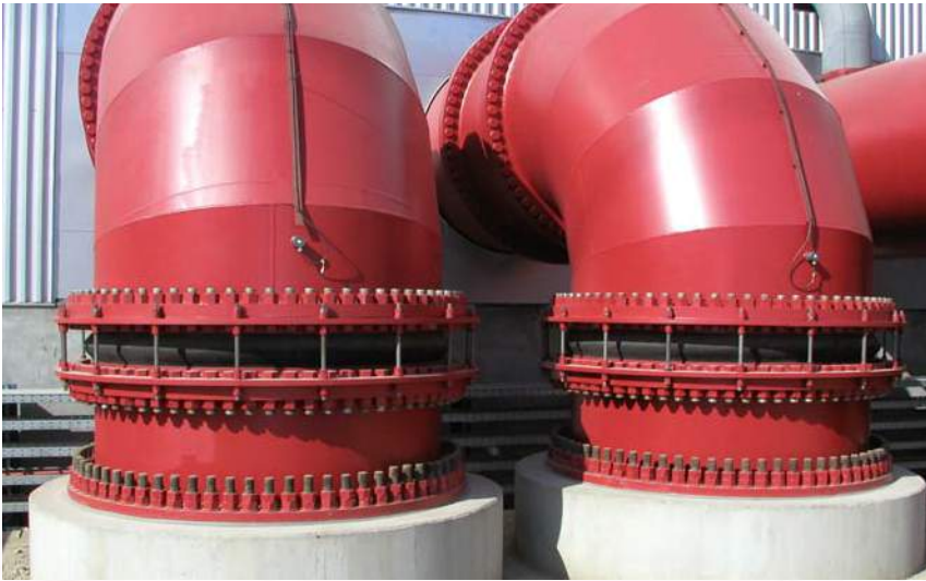
Very big expansion joints with tie rods on a power plant
