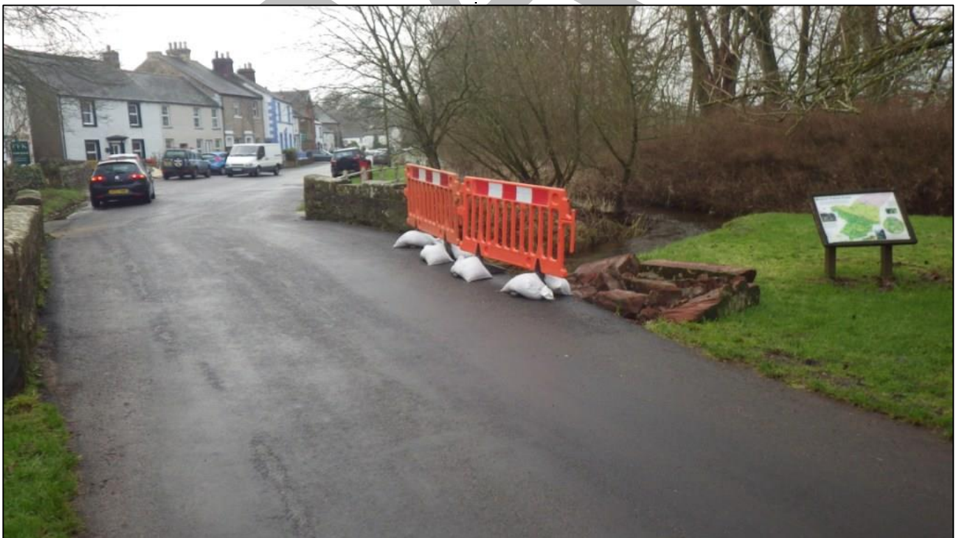
Photograph 3: Extent of damage on Warcop Bridge looking downstream 5 th December 2015, no timestamp
