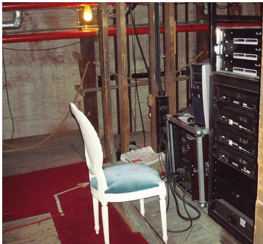
Het Toneelhuis' young technical staff is confronted by old technology for which adequate training no longer readily exists. The extensive chariot and pole system, traps, and old fly loft have all become obstacles in their states of neglect.
