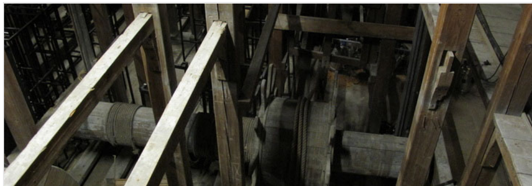
Original wooden structure and machinery on the two lower levels under the stage
