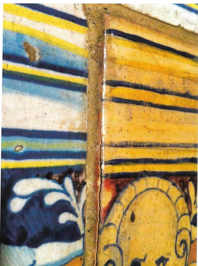
Figure 10. Detail of delamination of the polyester top layer (Copyright Melissa Vandevijvere)
