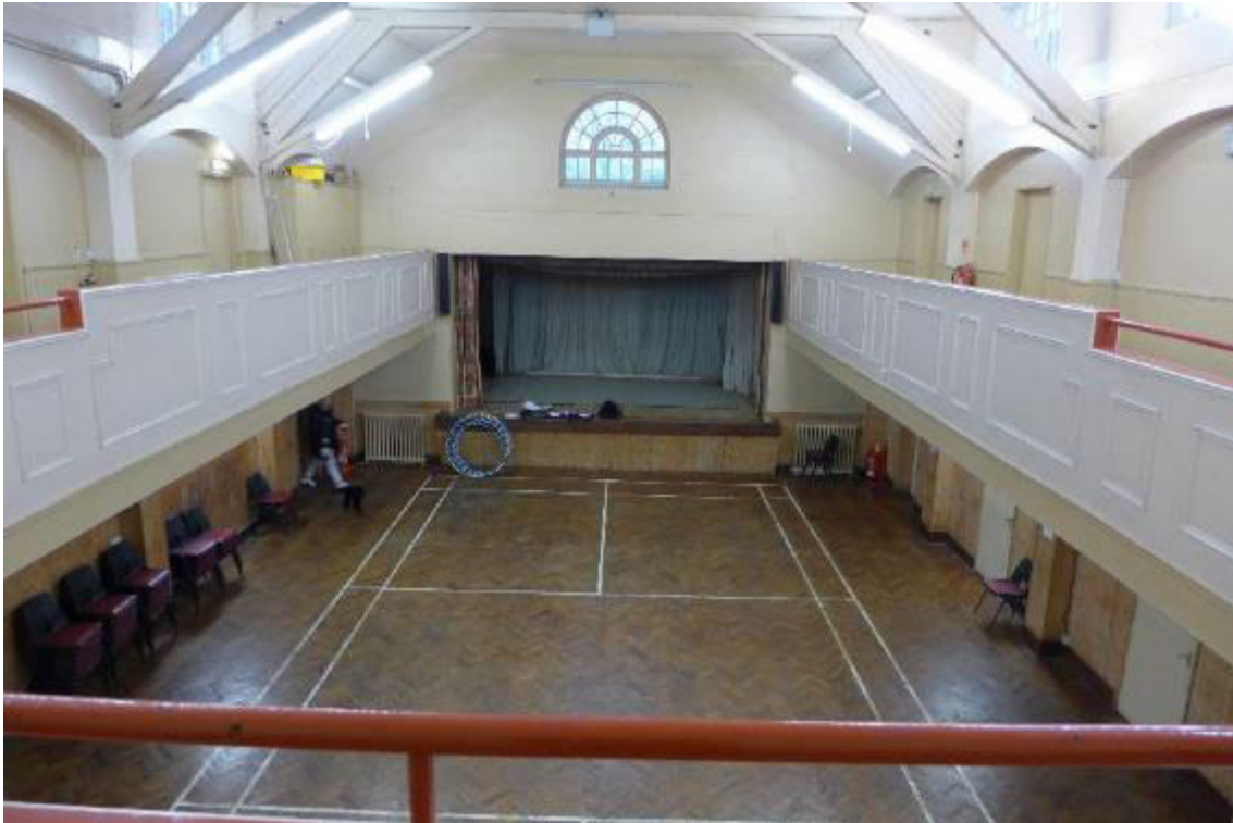
Fig. 49: The central hall looking east, showing the alterations undertaken in 1960/61 to create a new recessed stage. The gallery rail dates from the mid-1990s. (© Emily Cole)
