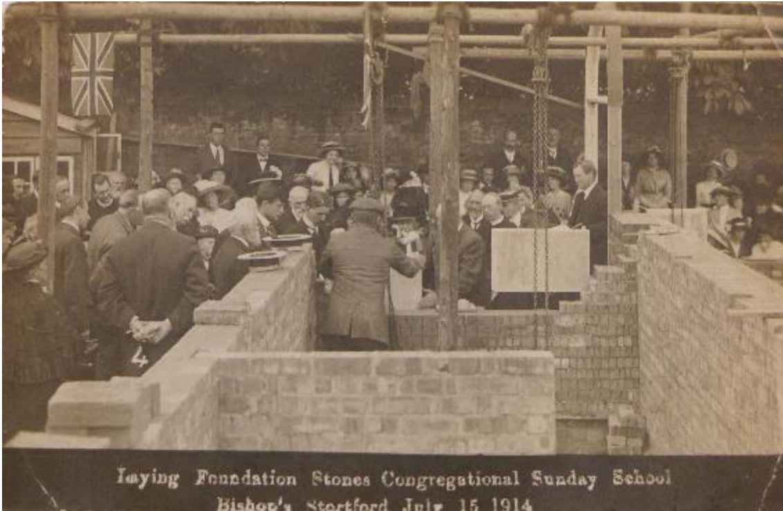
Fig. 7: The ceremony celebrating the laying of the foundation stones at the new Sunday School in Bishop's Stortford, 15 July 1914 (looking north). (Courtesy of Tony and Margaret Trigg)
