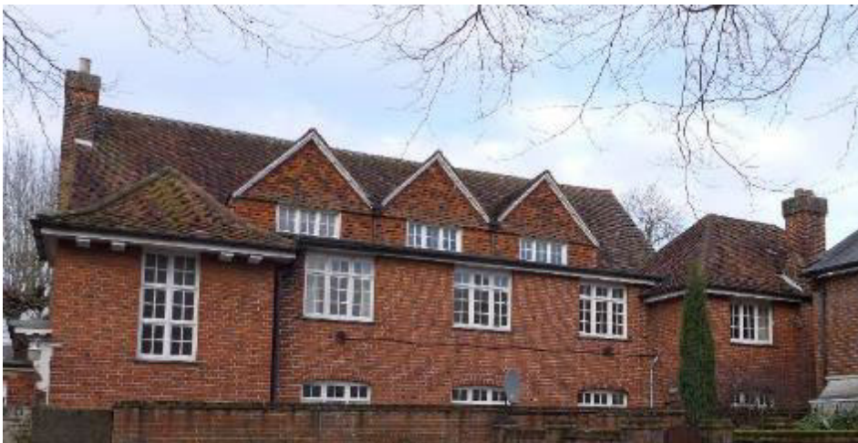
Fig. 31: The Hall from the south, showing well-preserved features including clay tiles, dormer windows with tile-hung gables above, eaves brackets, windows and chimneys. (© Emily Cole)
