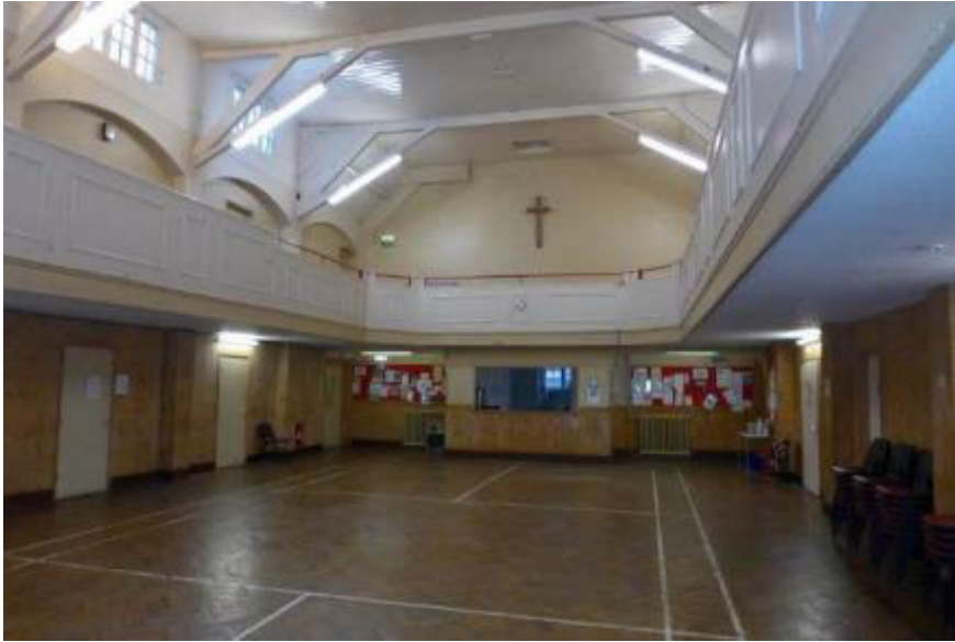
Fig. 50: View of the main hall, looking west. The present gallery edging dates to a reworking of 1994, but the original balusters apparently survive within. (© Emily Cole)
