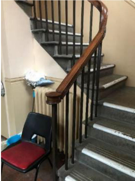
Fig. 59: The north-west staircase, which like the staircase at the south-west survives in unaltered form. (© Emily Cole)
