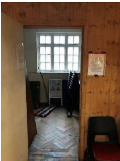
Fig. 47: View looking south into one of the former small classrooms opening off the ground floor of the main hall. (© Emily Cole)
