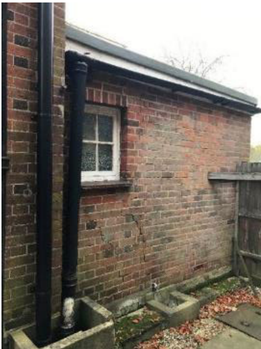
Fig. 37: The single-storey section of the south-east pavilion, showing the area of original brickwork (in the area of the window) which once supported a balcony above. This block was altered and extended in the 1930s. (© Emily Cole)
