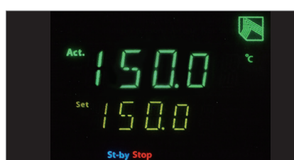
Clear VFD Controller.
