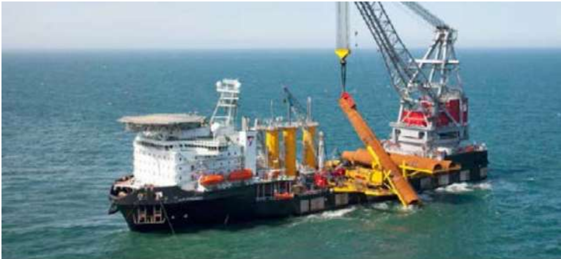
Heavy Lift Vessel (HLV). A heavy lift crane vessel lifting monopile foundations into place. The HLV utilizes dynamic positioning rather than an anchoring system to hold its position during installation.
