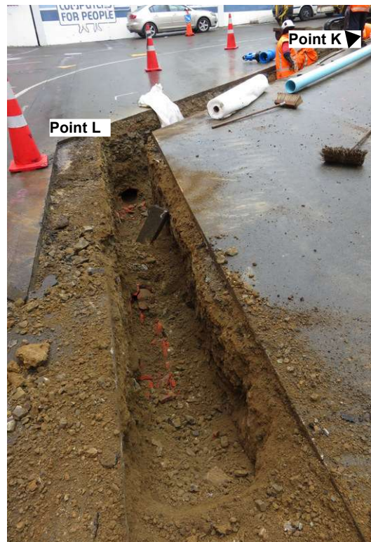
Illustration 27: Wide-bore red earthenware stormwater pipe Point L-Point M facing south-west (22 nd September 2015)
