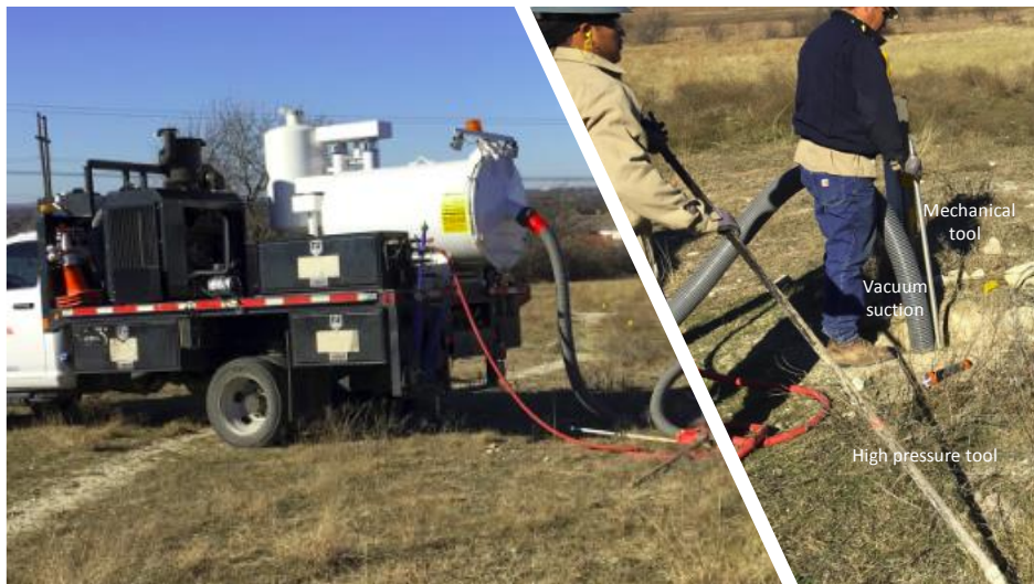
Local digging - air vacuum procedure involving high-pressure- and mechanical tool for soil release and a vacuum suction hose for removing the soil. (Photos with kind permission of Kantex).
