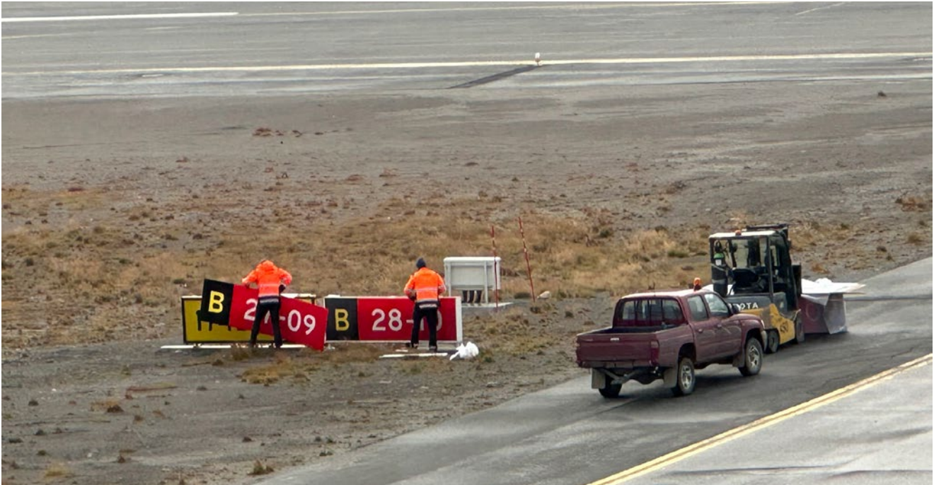
Figure 6: Runway signage at Longyearbyen airport being revised due to changes in the magnetic field. In September 2023, the old runway sign 28-10 (i.e., close to magnetic orientations 280^\circ and 100^\circ , respectively) had to be replaced by 27-09 ( 270^\circ and 90^\circ magnetic orientation) due to the moving magnetic pole. (Photo: Ine Therese Pedersen)
