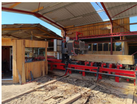
The association has taken over an existing family sawmill and installed a new electrical mill.
