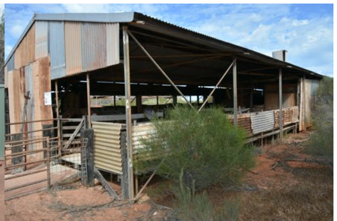
The salty winds take is toll of steel
