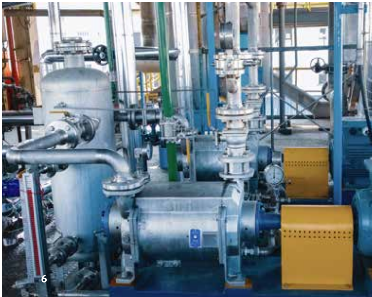
Two water ring pumps connected in parallel as atmospheric stage for venting
