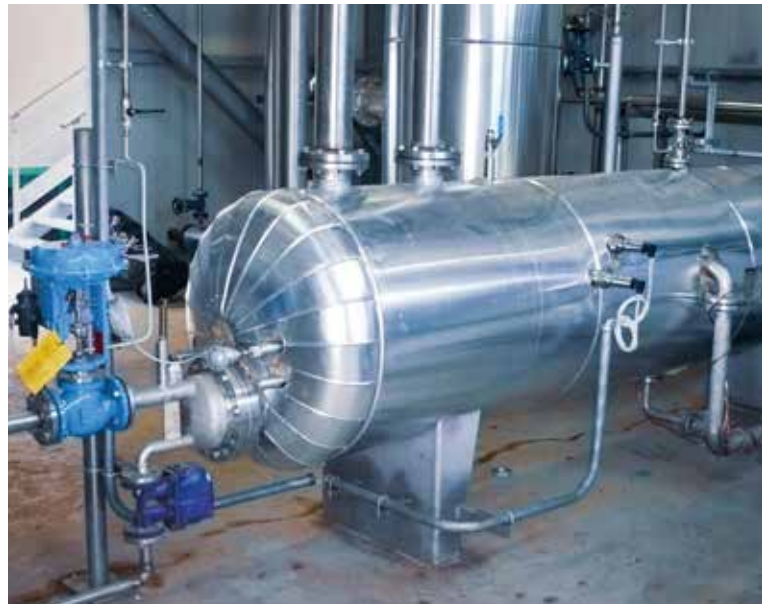
Melting vessel of a Körting ICE Condensation Vacuum System
