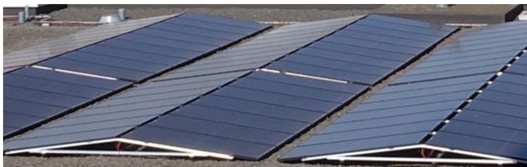
Figure 5 - Example of solar PV installation on a flat roof (orientation towards east/west)
