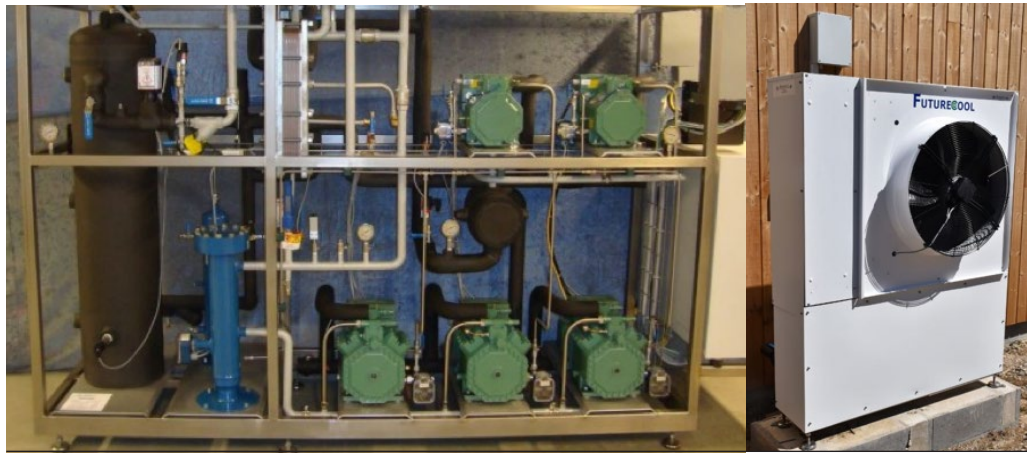
Figure 49 - Example of CO 2 cooling installation. Indoor unit (left) and outdoor unit (air cooled condenser) (right). Source: JF køleteknik A/S
