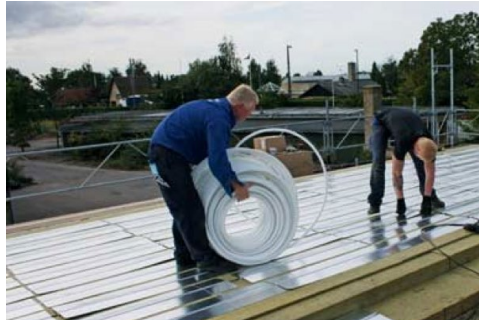
Figure 33 - The hoses for heat pumps in the roof construction [1]
