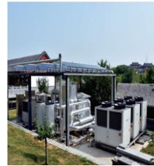
Industrial heat pump
