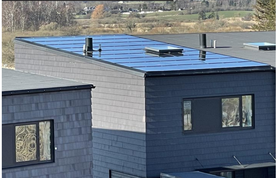
Active Roof with roof-integrated PV panels in Værløse, Denmark, from the private house of Peder Vejsig Pedersen
