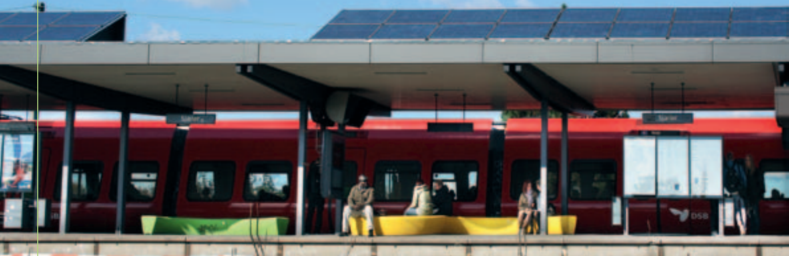
Train station in Valby - PV modules supply energy for the platform LED lighting.
