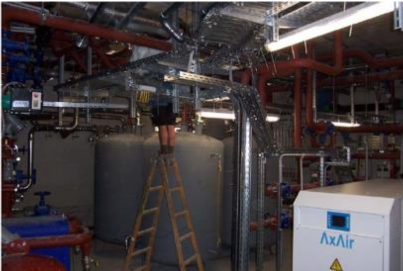
View of the district heating plant in the basement of the housing area
