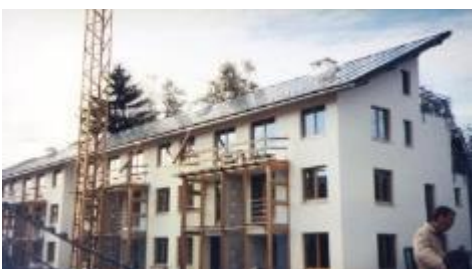
The European Green Cities partners also visited a new solar low energy project in Salzburg Gneis Moos, which made the first experiments with large communal solar thermal collectors together with a buffer storage tank connected to the district heating.
