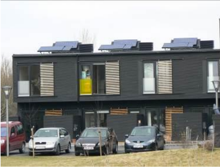
Karens Minde. The picture shows the installed photovoltaics in detail. One panel is placed on the skylight (the boxes) and the other photovoltaics panels are placed directly on the roof in a montage system with a slope of 30°.
