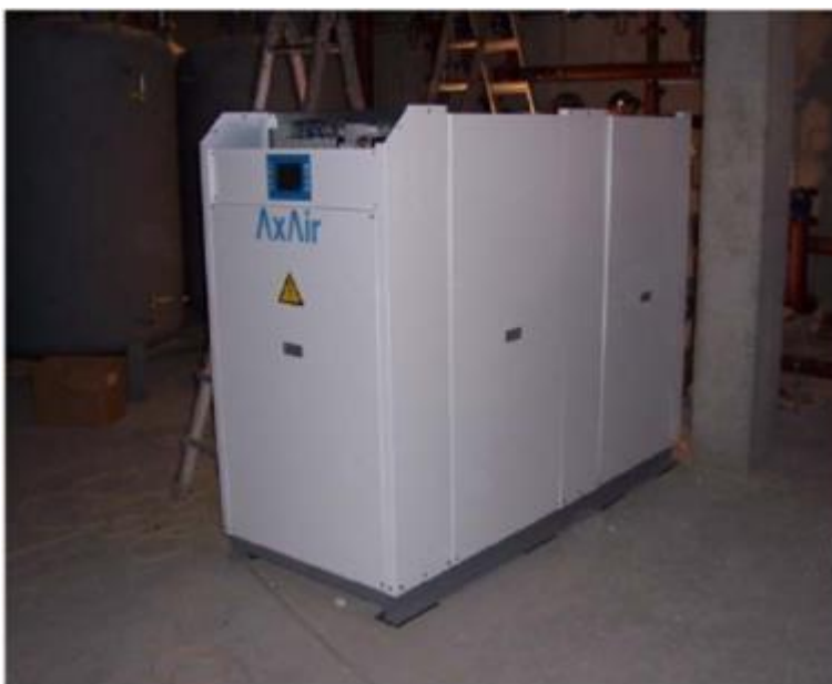
Electrical Heat Pump, nominal heat output 170 kW
