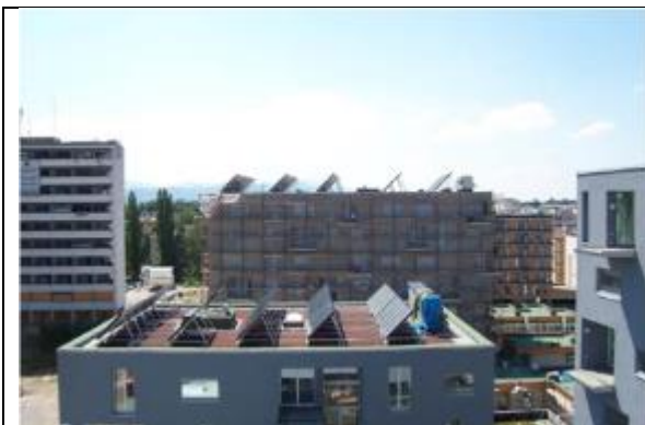
View of the buildings H and F with installed collectors and the ventilation unit on the north
