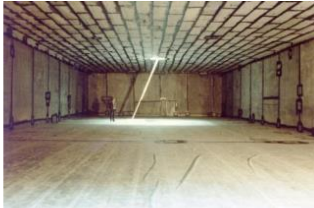
3.000 m 3 seasonal storage in Herlev placed under the solar collectors.
