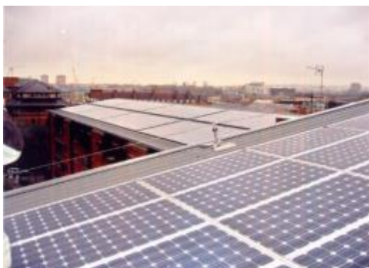
Example of PV implementation project in London by the Peabody Housing Trust and supplementing funding from the EU
