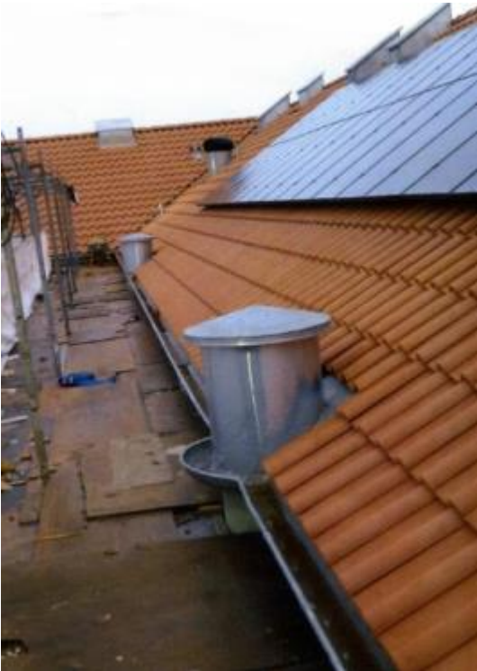
Example of a PV project from early 2013 in Valby Copenhagen in connection to a roof exchange project. Here the normal tile roof is exchanged first and later PV panels are mounted on top of this.
