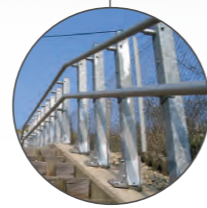
Rail for columns
