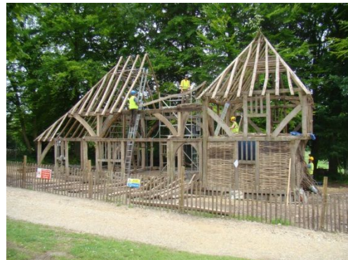
Sole Street, a medieval aisled hall from Kent, England, being re-erected at the Weald & Downland Living Museum, West Sussex, the latest timber-framed structure to join the museum's collections relating to historic buildings and rural life, which is Designated by the UK Government as of national and international importance
