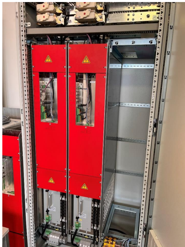
Figure 4: Typical installation in cabinet
