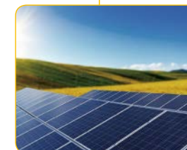
Solar power station
