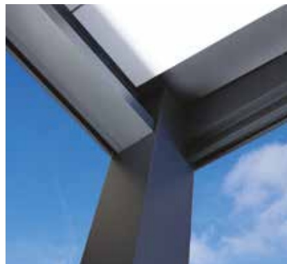
Waterafvoer via goot direct in steunpaal
