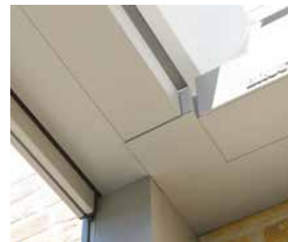
Waterafvoer via goot direct in steunpaal
