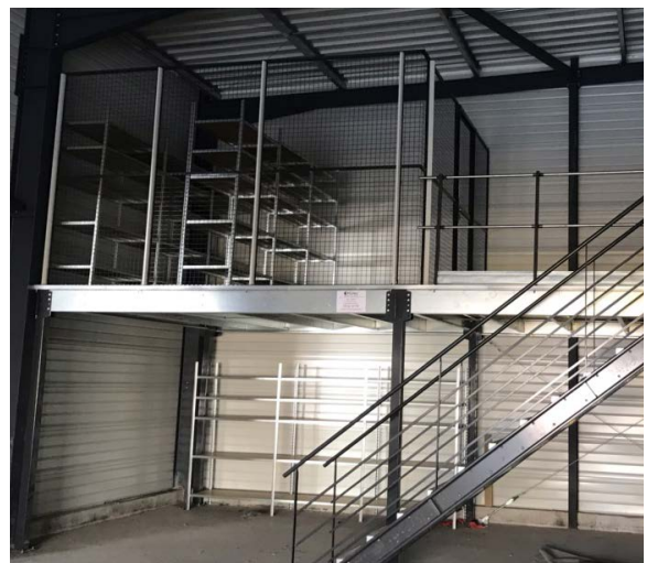
Delimitation of Adaptiv shelving using industrial partition wall, accessible via a Mezzaman Stock mezzanine.
