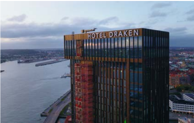
The new Hotell Draken will be Gothenburg's tallest hotel. PE is the main designer of the project, on behalf of contractor K21. Through the construction document, we were also commissioned by UPB to design the building's frame.
