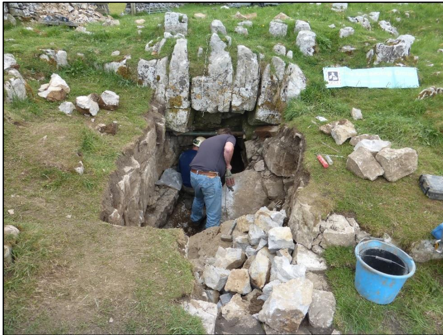
Tony and Luggie applying some rock engineering to allow insertion of the entrance pipe.
