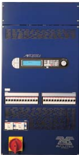
24 Channel Mainframe with Direct Circuit Connection
