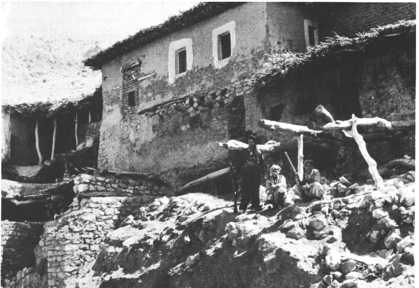
A bomb-damaged house at Galala.
