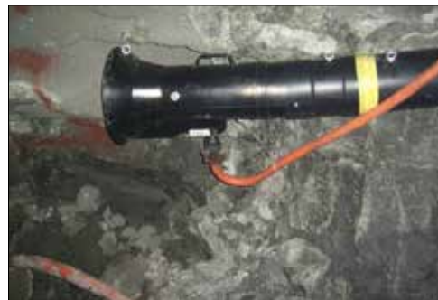
TERRAJET® Airmover Installed Underground
