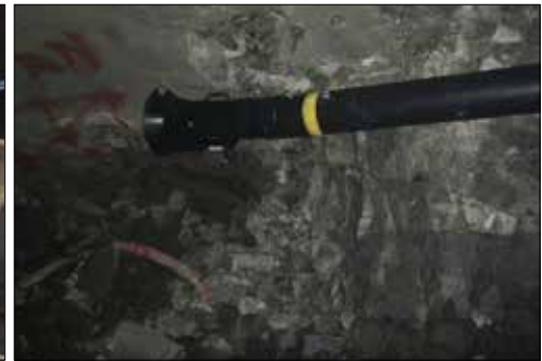
MK 3 Installed with PVC Pipe
