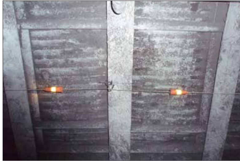
Escape Route Directional Cones installed underground with reflective tape
