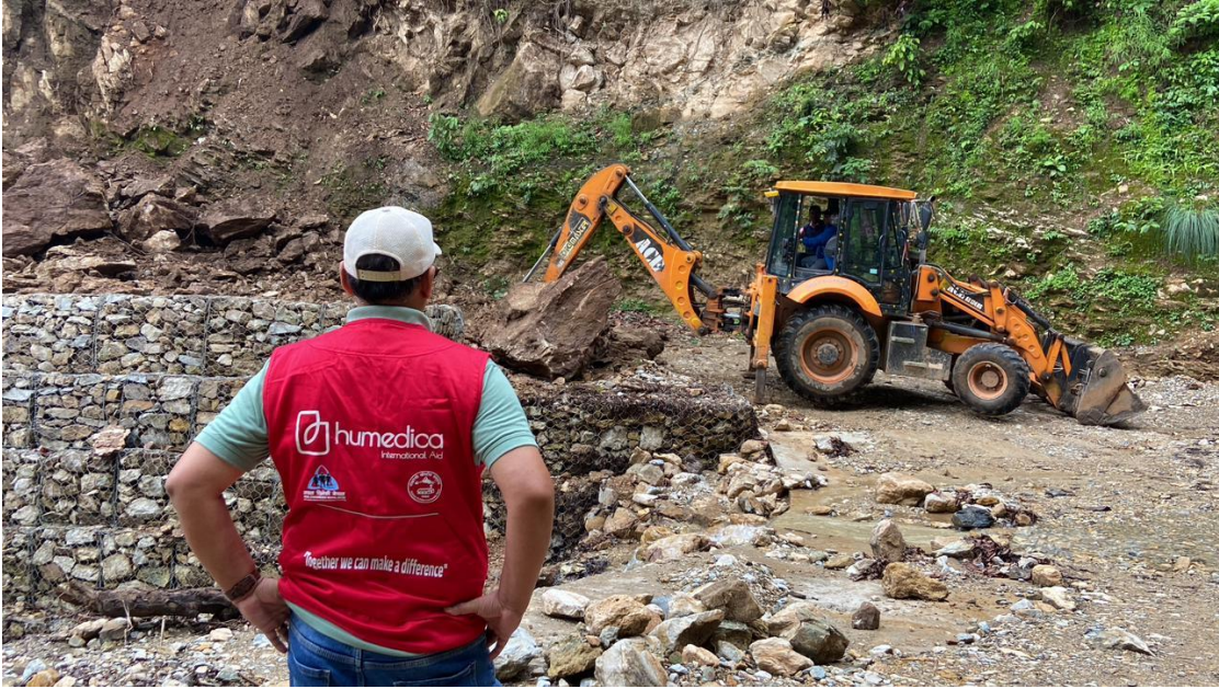
Road damages on the way to Rukkum.
