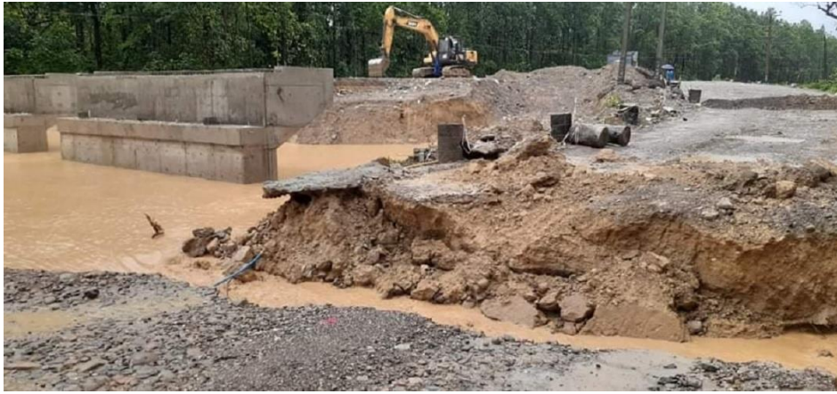
East-west highway, near Butwal, a bridge has been damaged and all movement has been halted.
