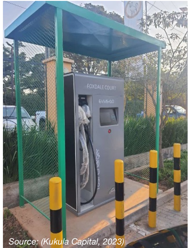
Figure 17: Foxdale Court's 60 kW fast DC EV charger
