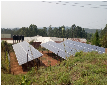
Current 25Kwp solarpower plant
