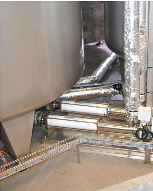
MIXING TANK ON LOAD CELLS AND PUMPING SYSTEM
