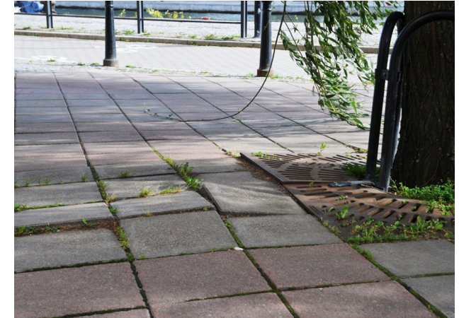
▲ Damage to pavement caused by roots due to inadequate volume of planting bed.
