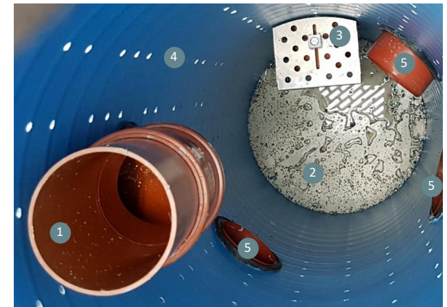
Control pit from above.
