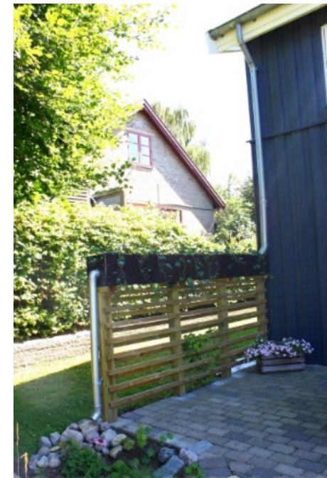
Figure 38 - the storm water planter in the back garden which is directly connected on the downpipes
