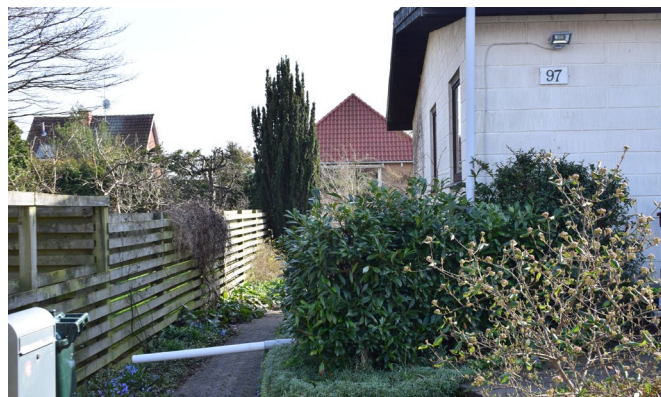
Figure 71 – documentation of efforts to divert rainwater from the roof into the flowerbed by the fence. However, this could create difficulties for the neighbours who could receive overflow as well
