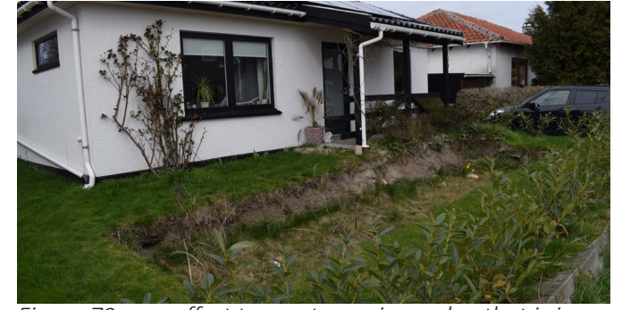
Figure 73 – an effort to create a rain garden that is in progress or unfinished
