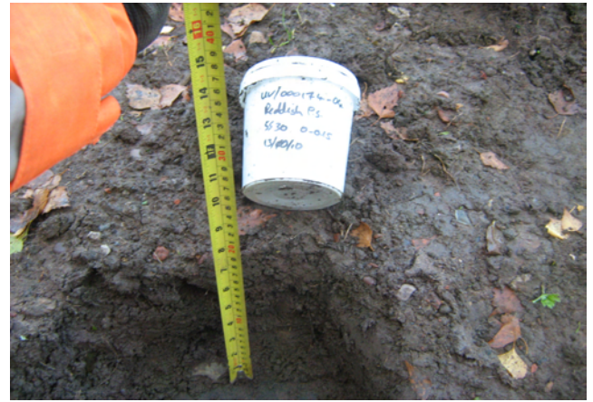
2. SS30 verification of subsoil depth - 150mm deep
