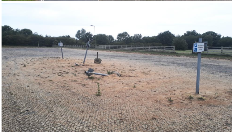
Figure 43. The park and ride site is in a poor state of repair
